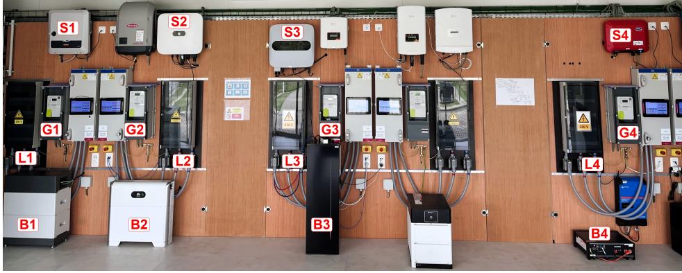
Figure 2.2: Photograph of the experimental setup: with G being the grid connection equipped with the official digital meter of the local distribution system operator, B the battery, S the solar PV installation inverters (solar panels equipped on the roof) and L the connectors to the dynamic loads (dimmers in separate cabinet and electrical loads stationed outdoors). The number represents the house numbers.
